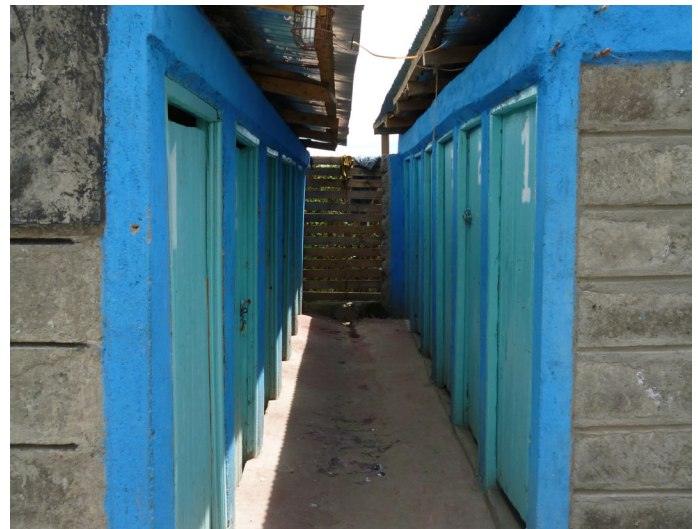
A recently upgraded shared toilet and bathroom facility in Nakuru, Kenya. Credit: Katherine Pasteur
