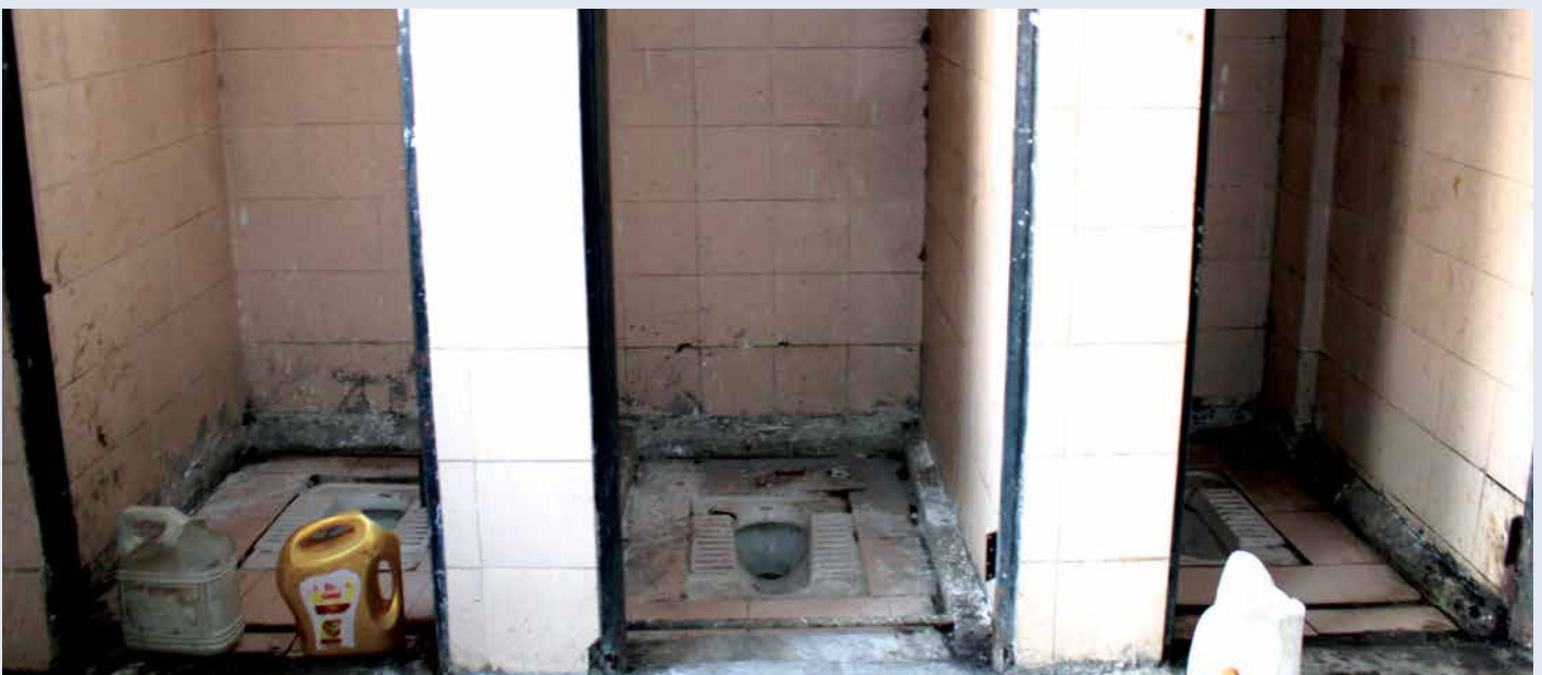
Pit toilets without doors, Pune. Photo credit: Lakshmi Anantnarayan
