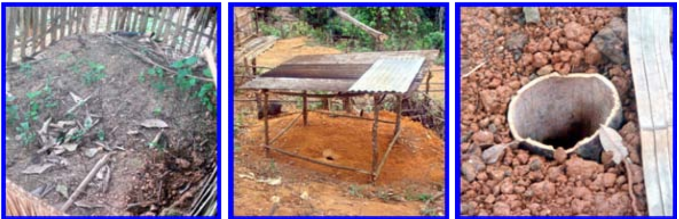
Some of the latrines not (yet) in use
