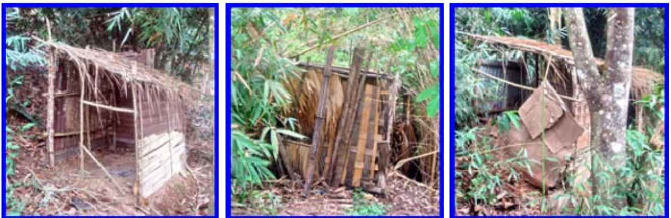
Dry pit latrines showing serious signs of fatigue
