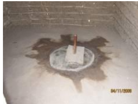
Fig 4: Improved traditional latrine
